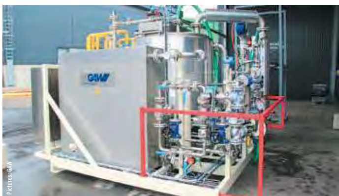
Mobile rental unit GAW starch preparation
