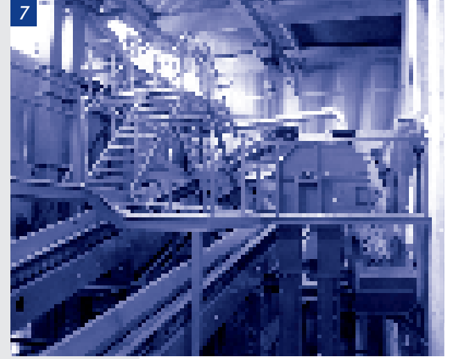
6/7 Industrial waste-treatment plant
